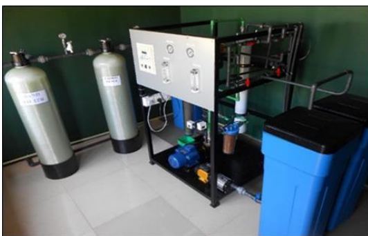
Figure 2: Brackish Water Reverse Osmosis Plant built by Sri Lanka Navy.
