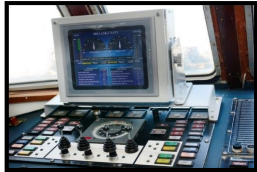
Figure 2. New Control and Monitoring Panel
