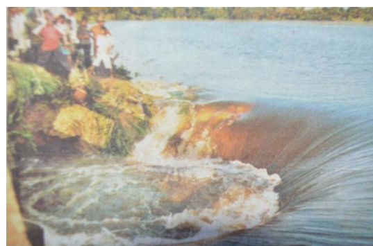
Figure- Damaged tank bund in Kidawaramkulama tan Source: Athula Bandara, 2004
