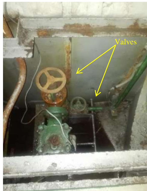
Figure 1: Bad valve placement in OPV-A
