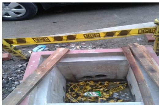
Photo 2: A newly constructed manhole has become a garbage bin!
