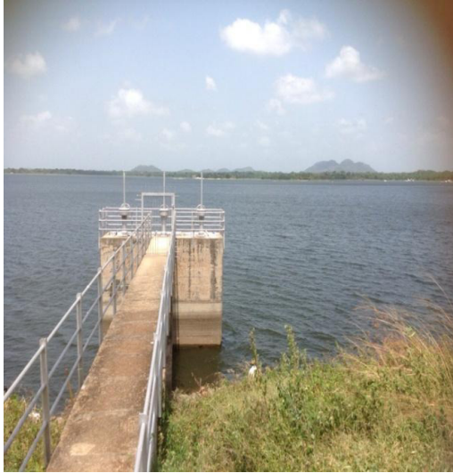
Figure 2: Sluice Gate at Rajangana Left bank
