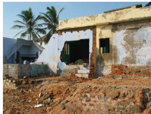
Figure 1: Failure of masonry Building against earthquake
